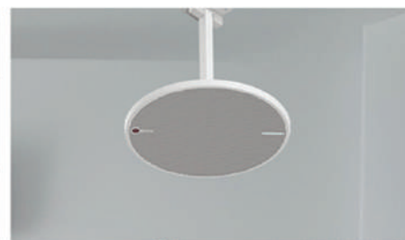
Installation with poles below the ceiling
